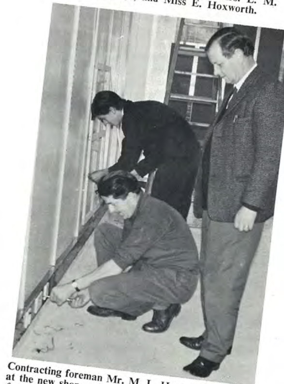
Putting the finishing touches to the electrical installation are Messrs. E. Naughton (electrician), left, and S. Larkin (apprentice).
